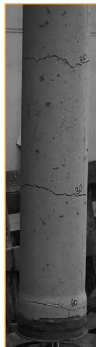
second crack (300 N/mm 2 )
