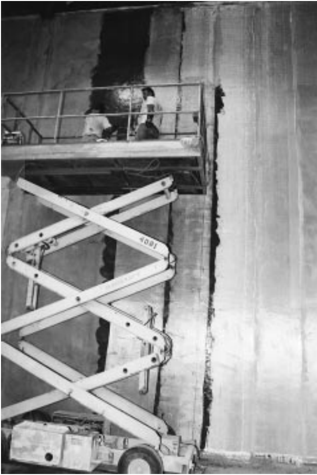
Fig. 8.17—Repair and strengthening of tilt-up concrete walls damaged during the 1994 Northridge earthquake
